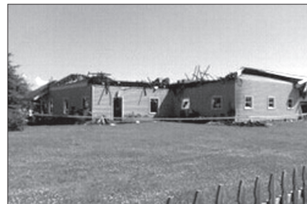
After the fire.
